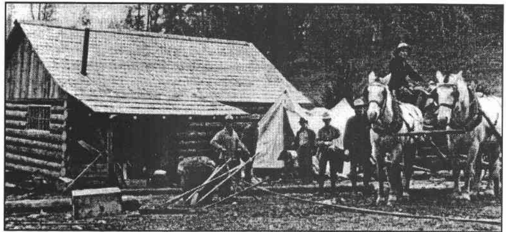
Figure 1-6. Rangers on the Sierra National Forest construct the Jerseydale Ranger Station in the early 1900's. Dolly and Dick, the Reserve's work horses, assisted.
