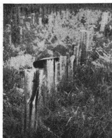
Split, black cottonwood posts given the hot- and cold-bath creosote treatment. No failures after 16 years, but tops are decayed. Top treatment was not given, but is shown to be needed.
