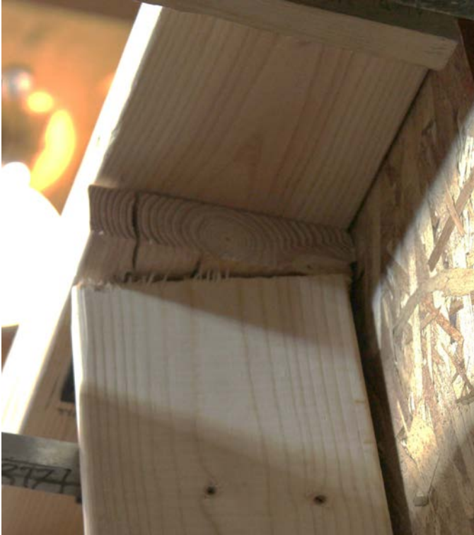
Fig. 11: Top plate splitting at stud connection
