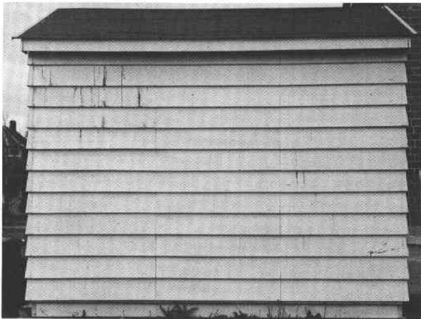
Figure 9. East wall of house covered with test sidings, after a year's exposure.
