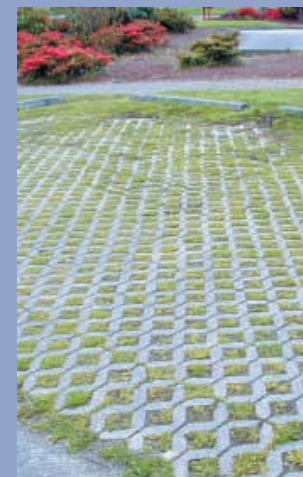
Permeable and porous pavements can reduce runoff, encourage infiltration, and filter pollutants. (Photo courtesy of Puget Sound Water Quality Action Team)
