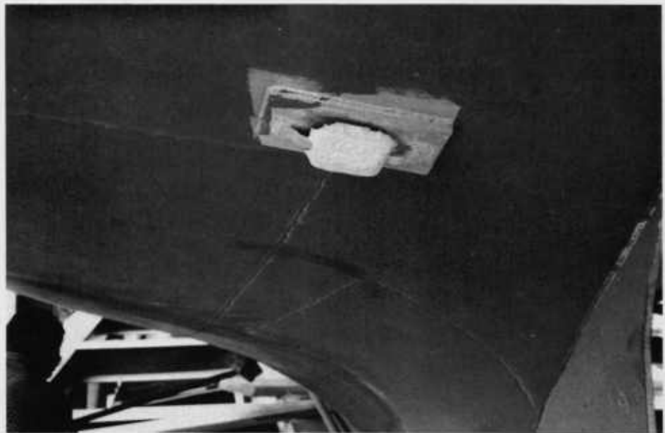
Figure 6.—A properly corroding zinc anode: (above) a closeup of the anode; (below) a fuller view of the hull area.
