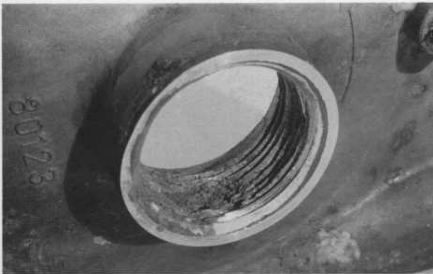
Figure 3.—The 1/4-inch stainless threads of this pump housing are badly corroded where a crevice was left between the housing and the threaded PVC pipe.
