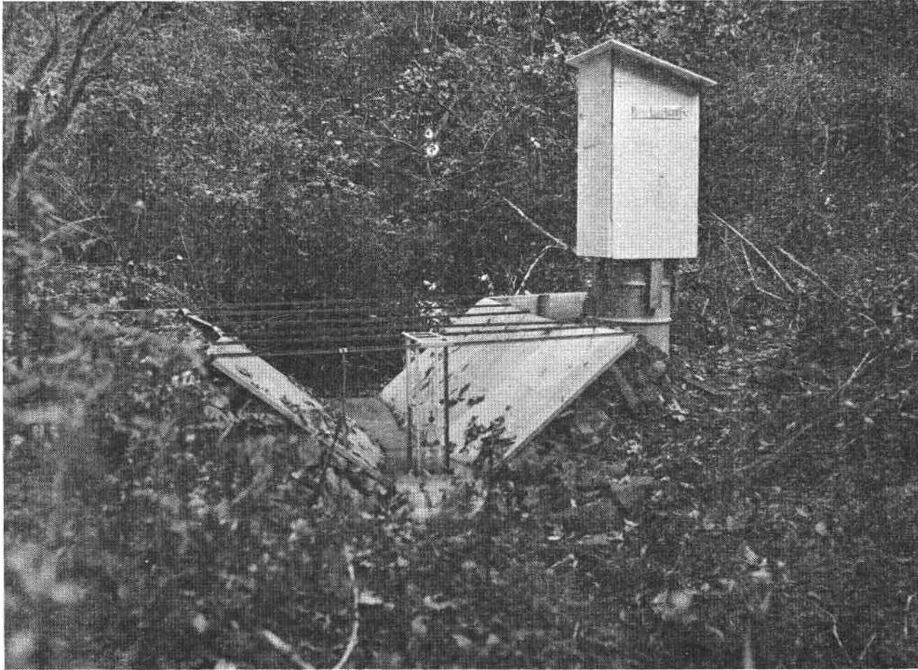
Figure 2. The gaging installation on Deer Creek II showing the flume, stilling well, and instrument shelter.
