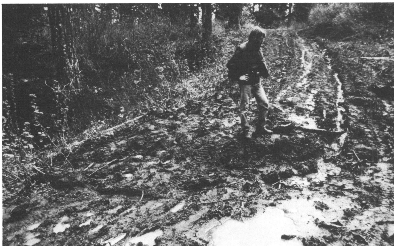
This rutted, poorly draining woodland road needs maintenance work.
