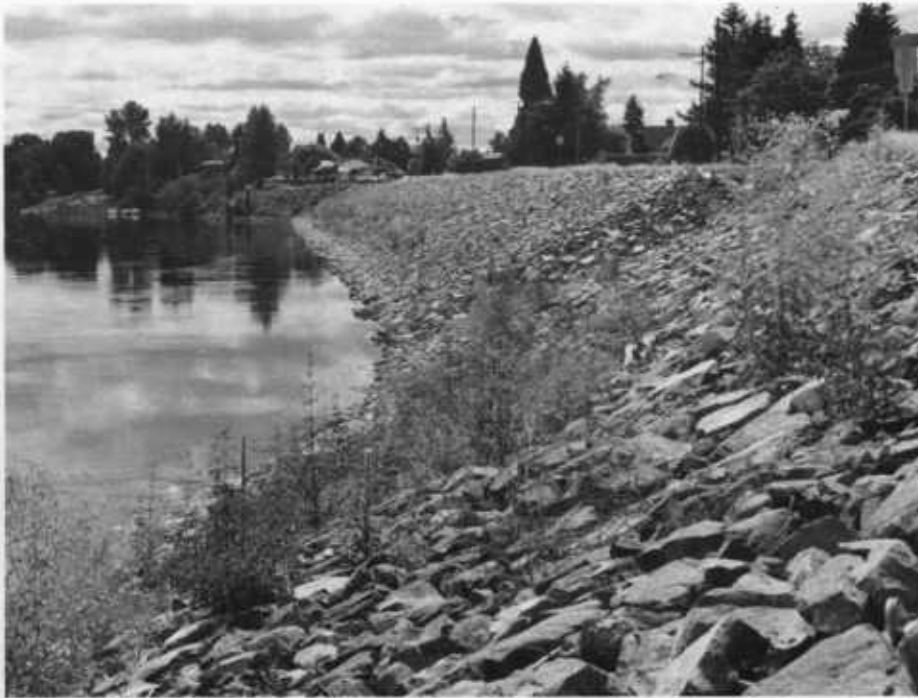
Riprap is a common streambank erosion-control method, but it may adversely affect both aquatic and riparian habitats.
