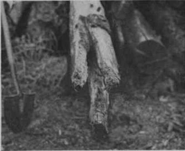
Salt-treated grand fir telephone poles in Gilliam County, removed after 10 \frac{1}{4} years because larger poles were required to serve an Air Base. Note characteristic distribution of the chemical in strips above and below the 3 bore-holes. Most poles here were sawed off at ground line.
