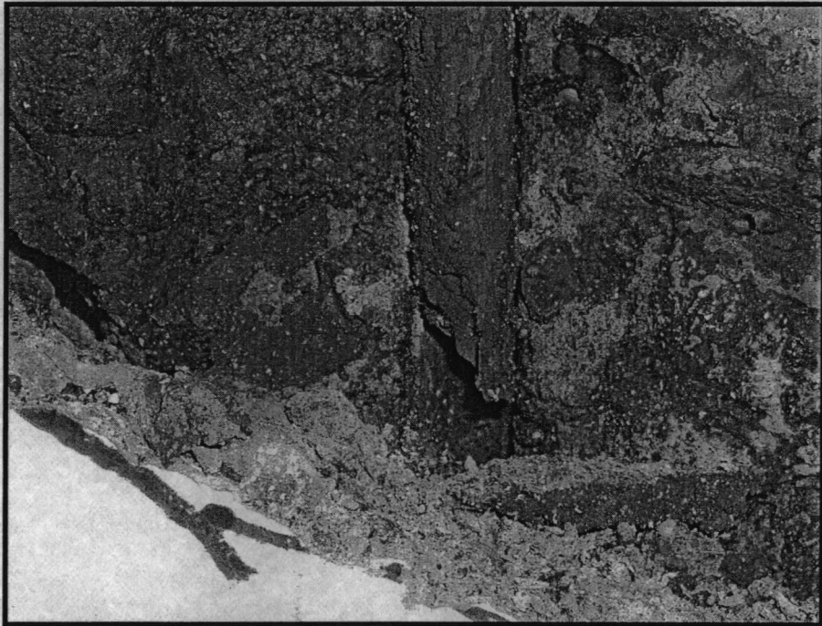
Figure 31: Completely corroded stirrup in bottom third of beam where shear crack formed.
