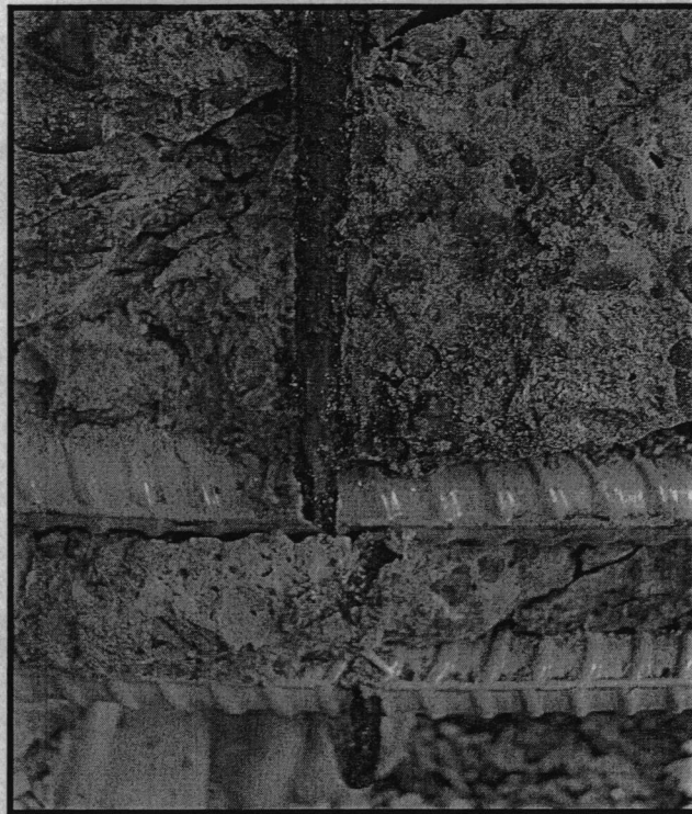
Figure 32: Fractured stirrup near flexural tension steel.
