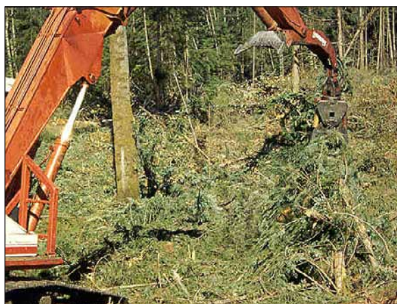
Figure 5.23. Place tops and limbs on the traffic lane and walk on harvest residuals before significant soil disturbance occurs, particularly on more sensitive soils.
