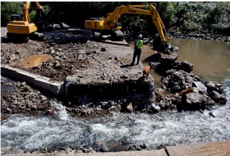
Figure 3. Brownsville Dam from the north abutment after the first stage of removal. Photo courtesy of John D. Martin, Cascade Earth Sciences
