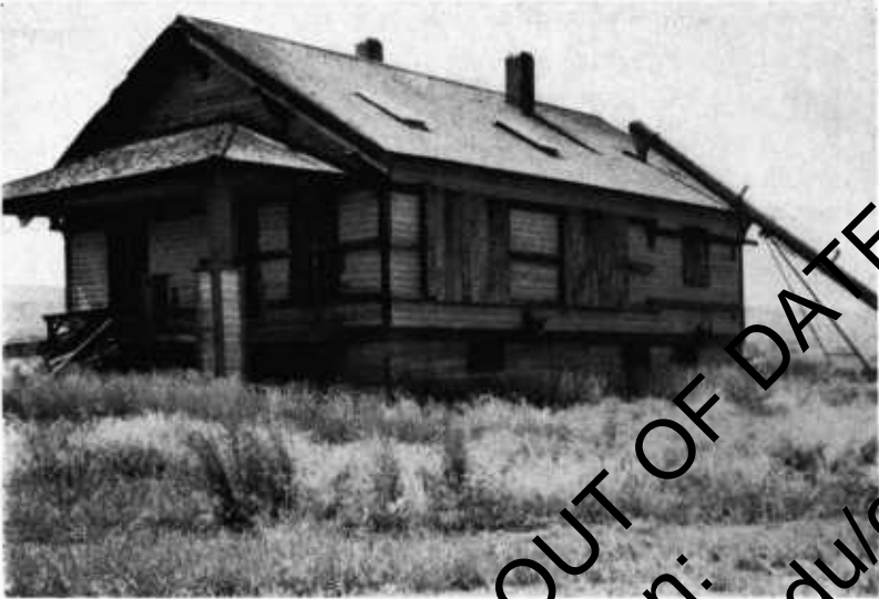
Figure 7. Using structures not intended for grain storage results in making exclusion of rodents and birds both difficult and expensive.
